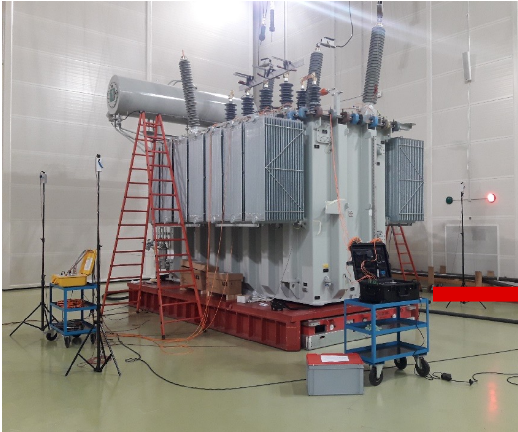
Transformer during Heat Run Test
