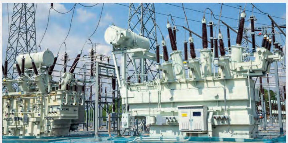
Figure 2. The complexity of cooling transformers has increased over recent decades resulting in higher efficiency and less noise emissions.
