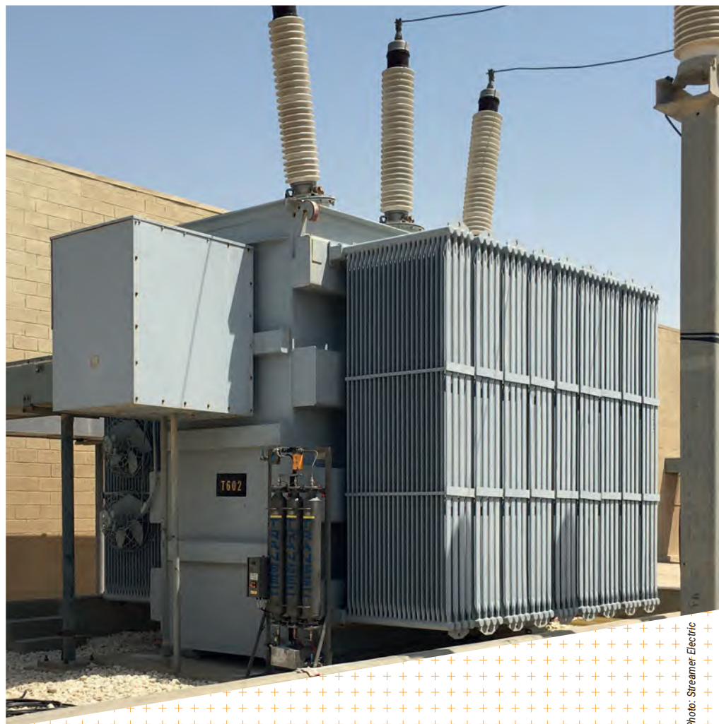
Figure 10. Online drying device with moisture monitoring installed on a transformer in Saudi Arabia's Abqaiq region
